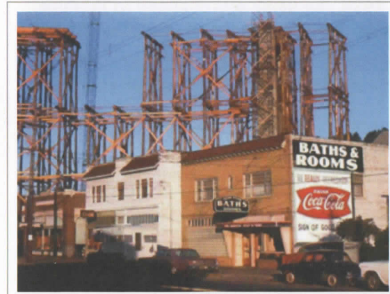
Finnish Meat Market, Worker's Club and Union Baths during construction of Astoria-Megler bridge.
